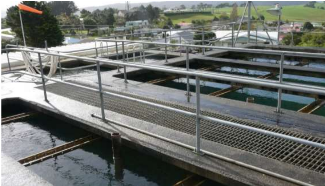
Figure 3-4: Dargaville/Baylys WTP clarifier
